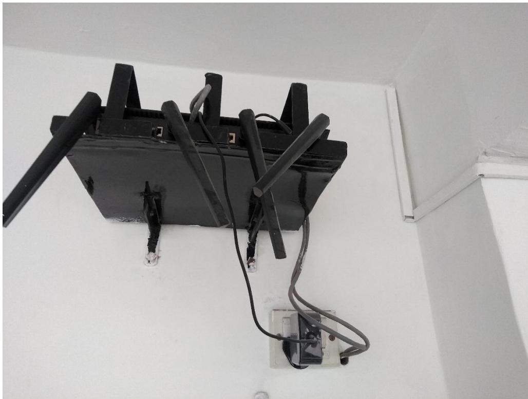
Servers and Wi-Fi Router
